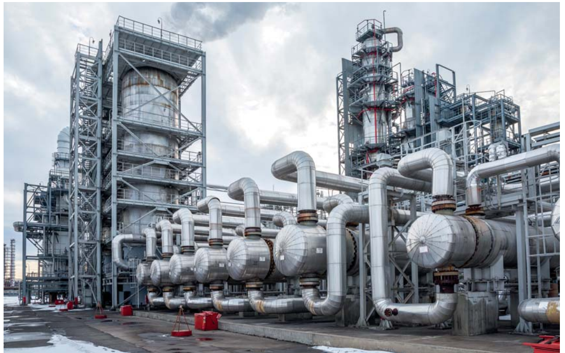
➤ Heat exchangers installed at an oil refinery. Source: Dreamstime
